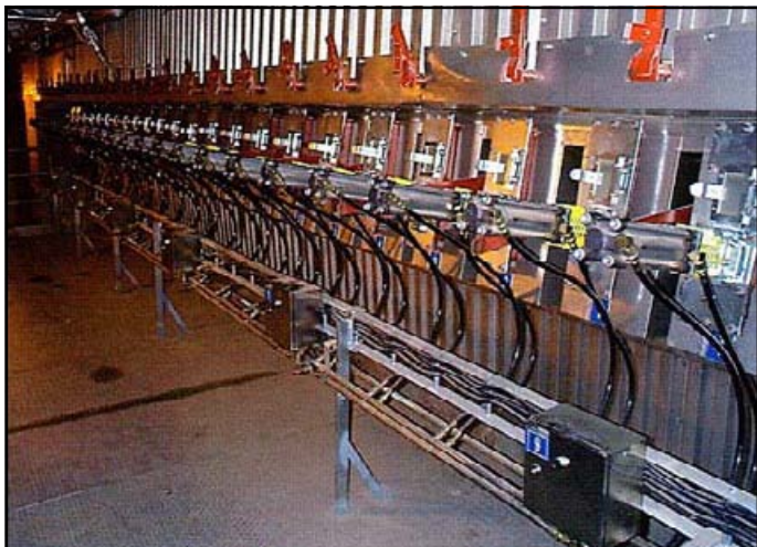
Installation of Diamond Rodding Robot on primary air level.
