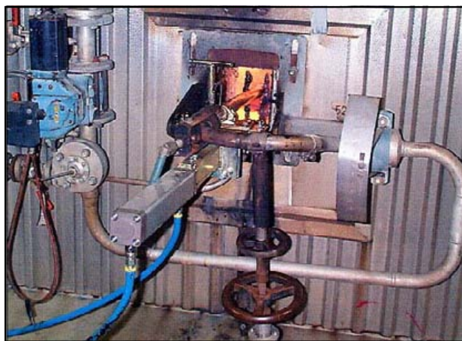
Installation of SPRAYROD for rodding of splash plate on black liquor gun.
